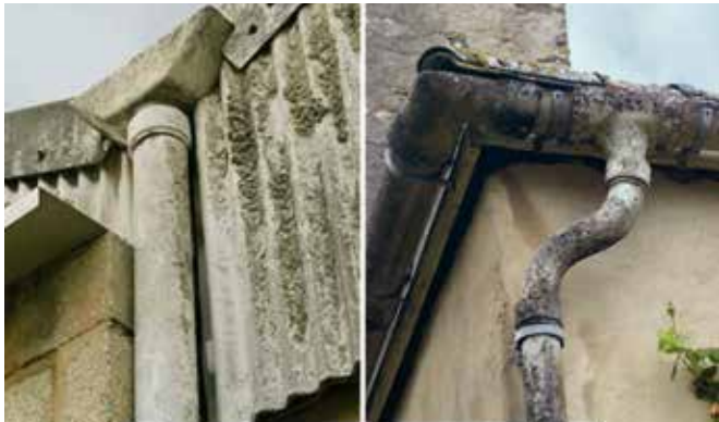
Asbestos cement downpipe and corrugated asbestos sheet
